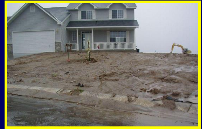
Poor Construction Practices
